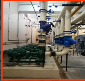
Mechanical & Pump System
