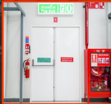
Fire Fighting/Fire Alarm System
