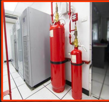
FM200 Fire Suppression System
