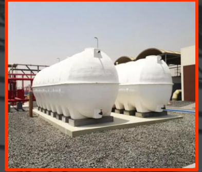
Water Tank & Plumbing System
