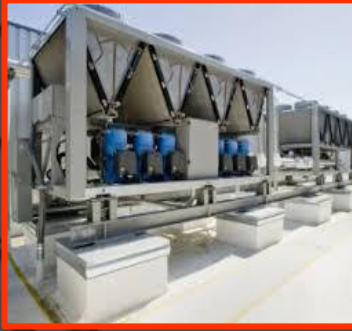
Heat, Ventilation & Air Conditioning System (HVAC)
